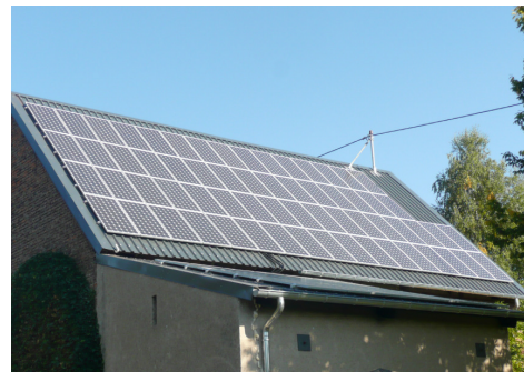
14 kWp Scheune in Gierschnach
